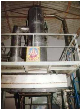
A 20 kW gasifier for rural electrification at Hanumanthanagar. It is a companion system for the system at Hosahalli. They are used for house illumination, drinking water supply and supply of irrigation water, and operating the hulling machine
